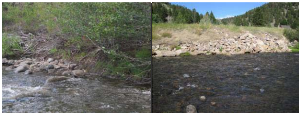
Figure 4-5. Typical eroding streambank conditions in Boulder River Reach 12-04.
