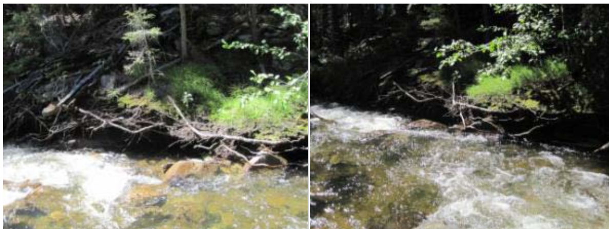
Figure 4-10. Typical eroding streambank conditions in Cataract Creek Reach 18-01.
