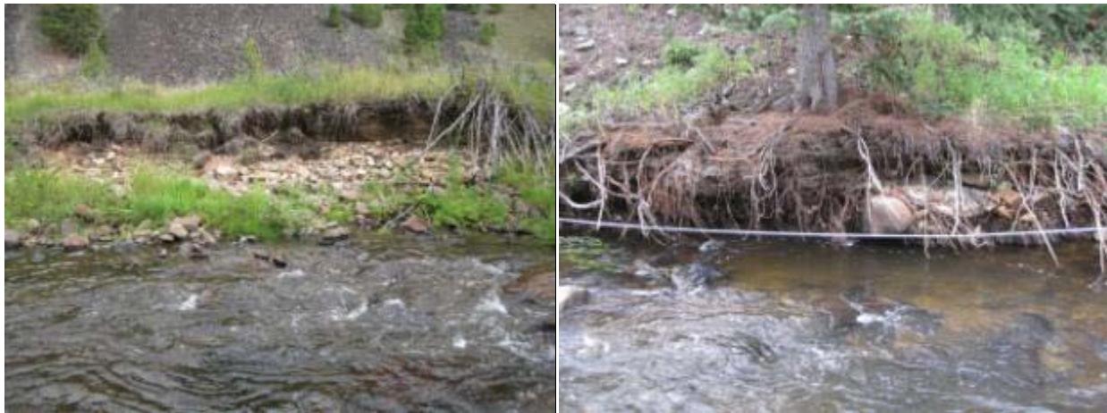
Figure 4-4. Typical eroding streambank conditions in Bison Creek Reach 11-01.
