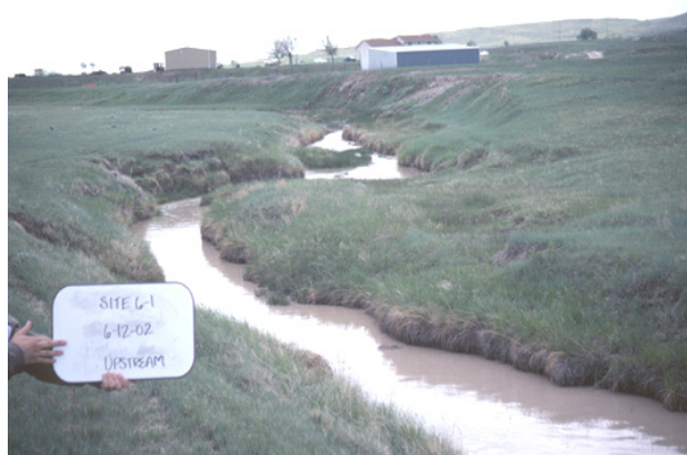
Lack of large woody vegetation and shade at Pumpkin Creek segment 6. (Photo by NRCS).
